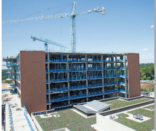
Construction of the New Sibley overlooking the green roof on the Radiation Oncology Center.
